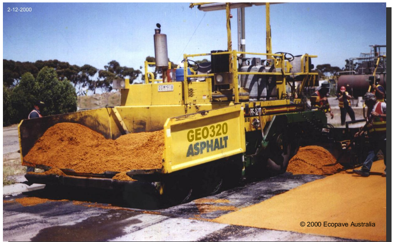
GEO320™ asphalt paver application at Melbourne Deer Park. Note the lack of fumes generated from the asphalt which was laid at 110°C (Warm Mix Asphalt).
